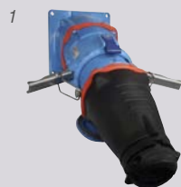
The plug is partially inserted, clamps are placed around bolthead, ready to pull the plug into the receptacle
